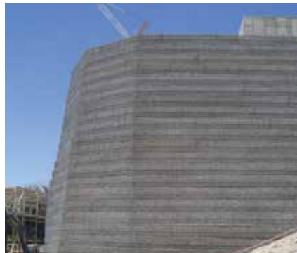
TXI Facility – Oro Grande, California
