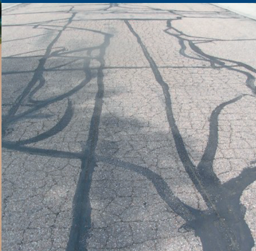
FILL MAJOR CRACKS
