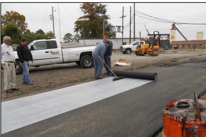
Figure 1 Installation of GlasPave fabric on a test section at East Alabama Paving.
