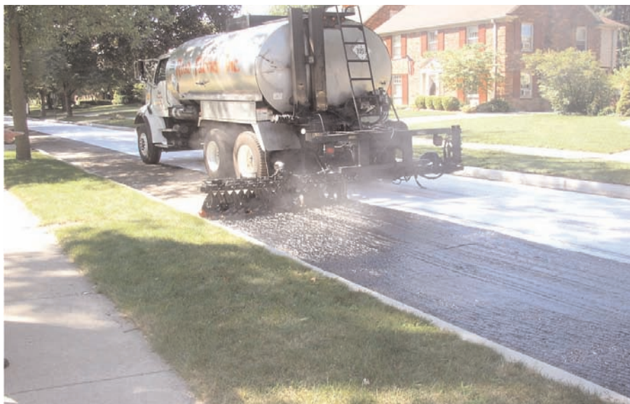
TruPave® installation, showing the application of hot asphalt tack and TruPave® installed on the adjacent lane. Hot asphalt tack also serves as a "crack filler" on small to micro-cracks on the existing surface.
