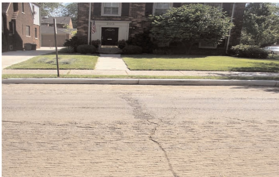
Photo taken in July 2006 as part of construction preparation of the asphalt wearing course showing fatigued pavement transverse cracking. Milled curb lanes were done to improve crown and slope corrections prior to paving.
