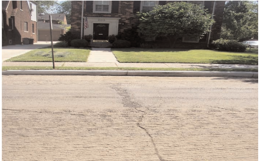
Photo taken in July 2006 as part of construction preparation of the asphalt wearing course showing fatigued pavement transverse cracking. Milled curb lanes were done to improve crown and slope corrections prior to paving.
