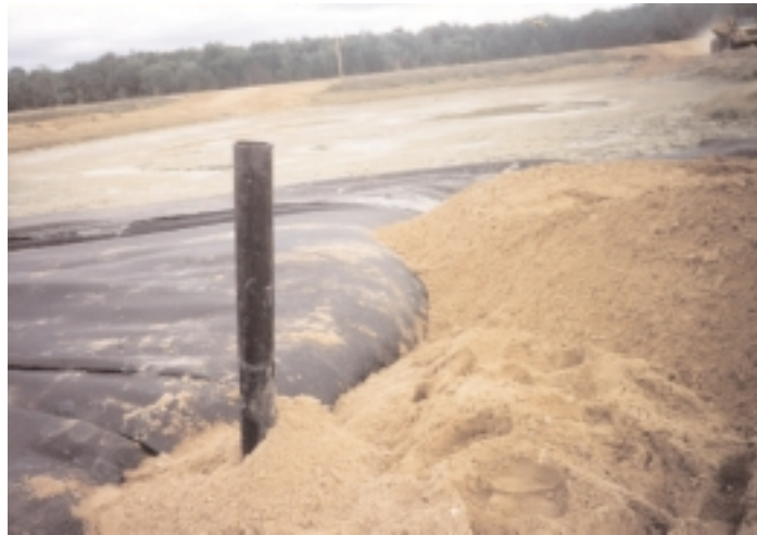
When ground displacement did occur, the geotextile stretched with the deformation of the sludge in a tensioned membrane effect.
