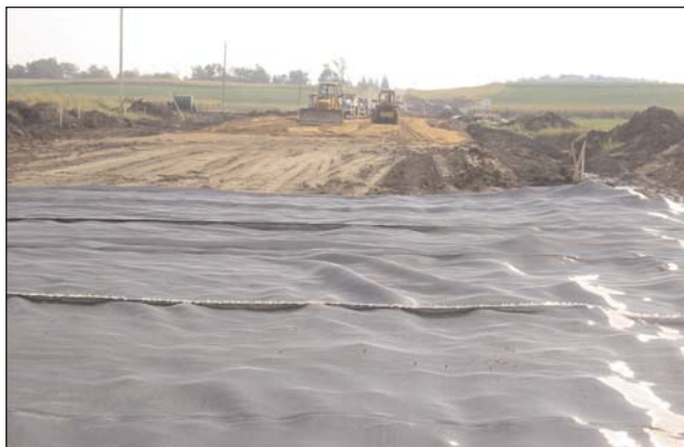
Due to the soft, peat subsurface, Geolon® HP770PET was required to complete the road widening project.
