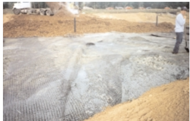
When ground displacement did occur, the geotextile stretched with the deformation of the sludge and split apart.
