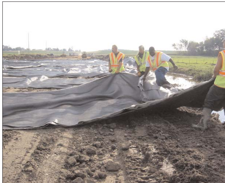
After the Geolon® HP770PET panels were seamed together, 3m (10ft) of fill soil was installed and left for 4 months to compact the excess pore pressure of the peat.
