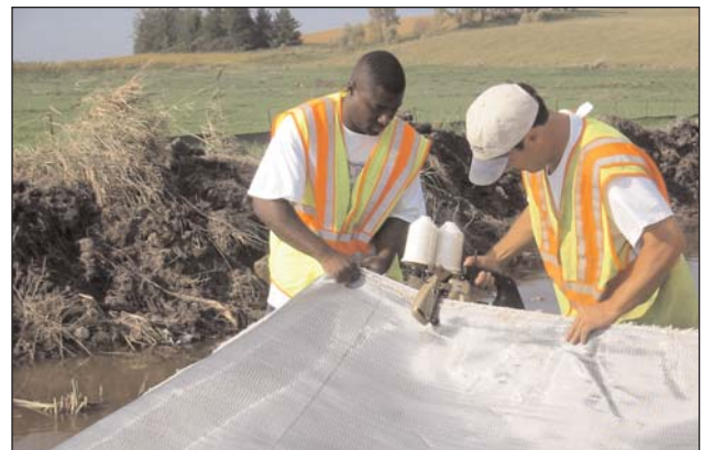
Overlapping the fabric would allow the mud to move up between the panels. Seaming was required to maintain 100% coverage.
