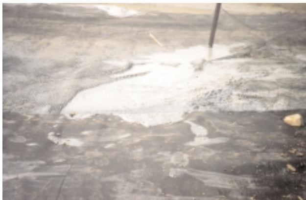
Geolon® HP665 prevented sludge from flowing up through the geotextile, the geogrid did allow the contaminated mud to soak through into the overlying fill.
