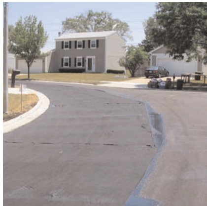
After the fabric is installed, pavement overlay was spread with 5cm (2in) of IDOT hot mix asphalt.
