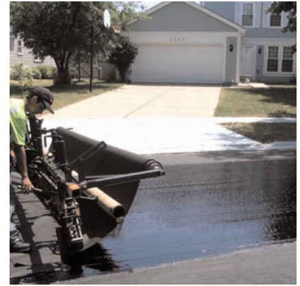
It is necessary to install the paving fabric in a timely manner when using a modified asphalt binder.
