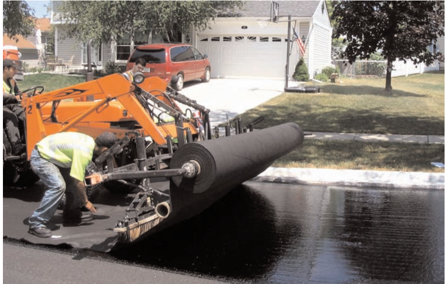
Mirafi® MPV 700 paving fabric is installed on top of the modified asphalt tack coat.
