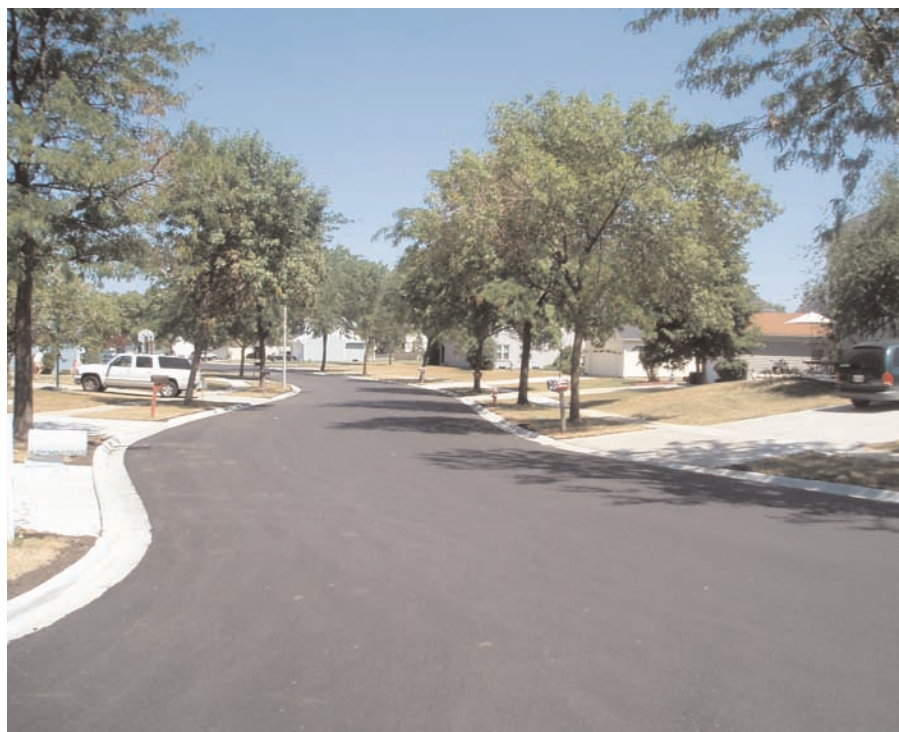
Thick paving fabrics such as Mirafi® MPV 700 are ideal for cold, harsh climates. The completion of Kensington Street with Mirafi® MPV 700 should delay reflective cracking.
