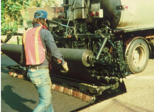
Figure 5: Distributor mounted equipment
